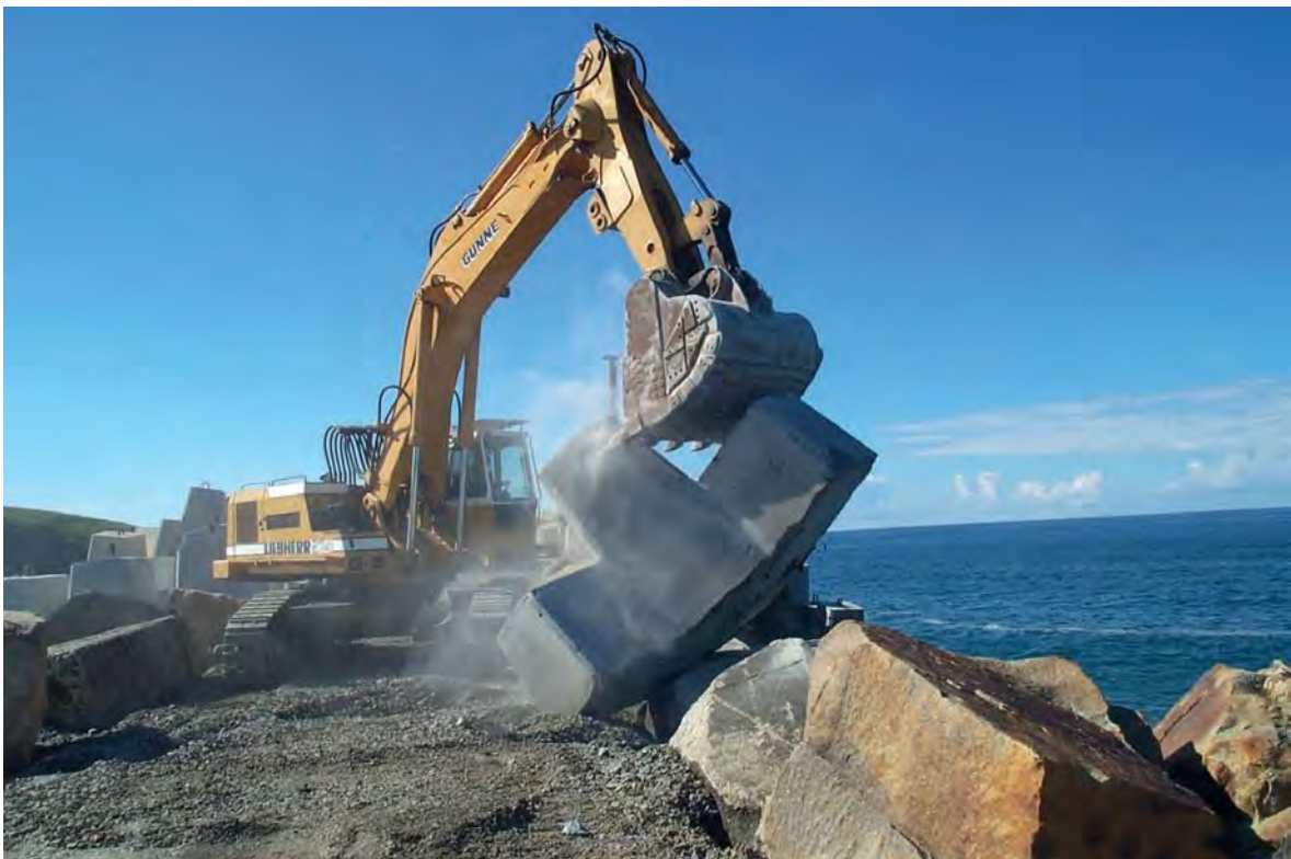
Coffs Harbour seawall repair with Hanbar units. SOURCE: NSW Manly Hydraulics Laboratory, Office of Environment and Heritage
