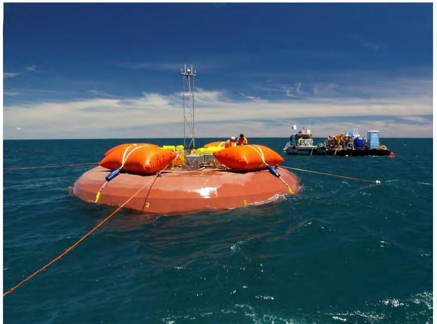
Carnegie CETO wave power generator installation off Garden Island WA Courtesy Carnegie Clean Energy Ltd
