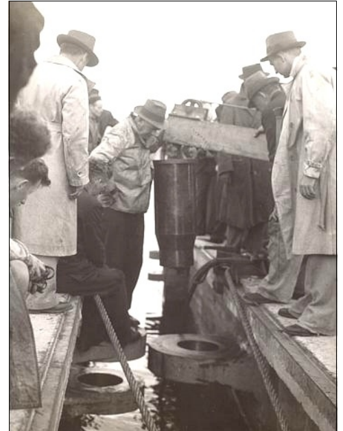
The centre pin holding the two half-arches together about to be installed.
