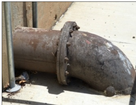
Cooling water pipe from the condensers. Photo KB
