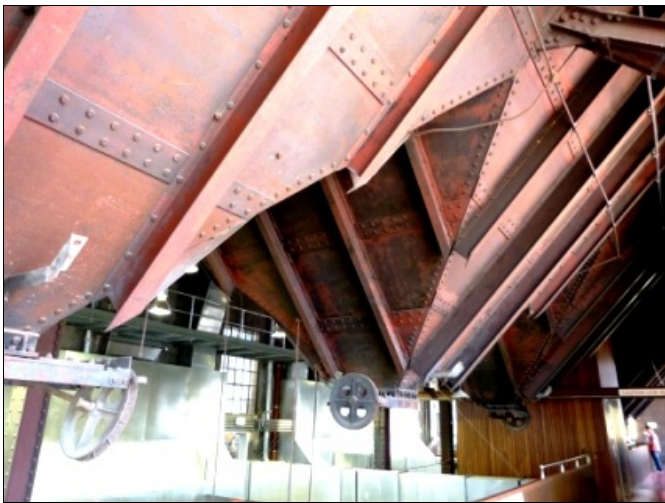
The retained coal hoppers hang above the Glass Hot-Shop in the former Boiler House of the Kingston Powerhouse. Photo: Keith Baker.
