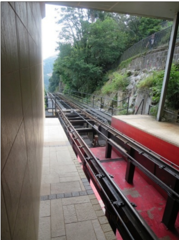
The cable for the down car (between the rails) is seen from behind the up car at an intermediate station. Empty rollers for the up car cable are visible outside the station. Photo: Brian McGrath
