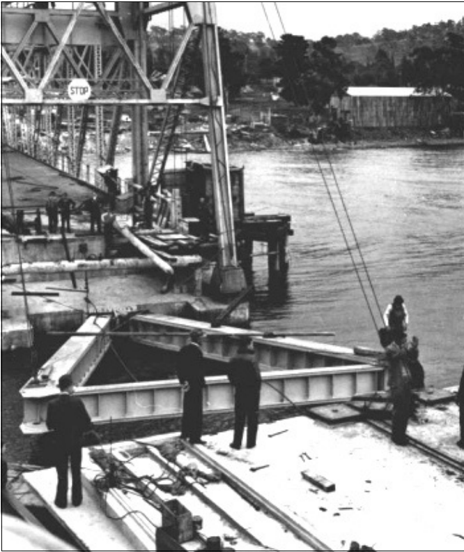
Connecting the triangular hinge frame to the concrete pontoon at the western abutment of the bridge (next to the lift span). Source unknown.
