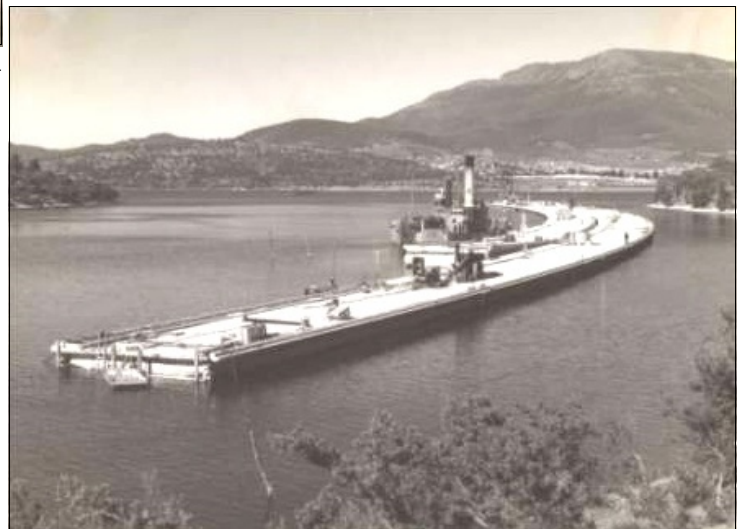
The two completed half arches parked in Geilston Bay. One of them is ready to be towed out into the river and moored to a buoy located where the apex of the arch would be.
