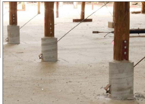
New concrete pole footings with shortened poles bolted to them & diagonal bracing rods passing through them. Photo: Martin Zweep, May 2011.
