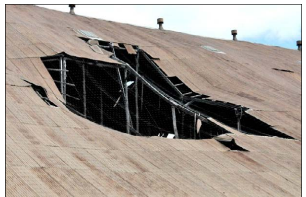
RIGHT: A large hole in the roof of the Stick Shed, seen in October 2010, before repair work started. Photo: Owen Peake.
