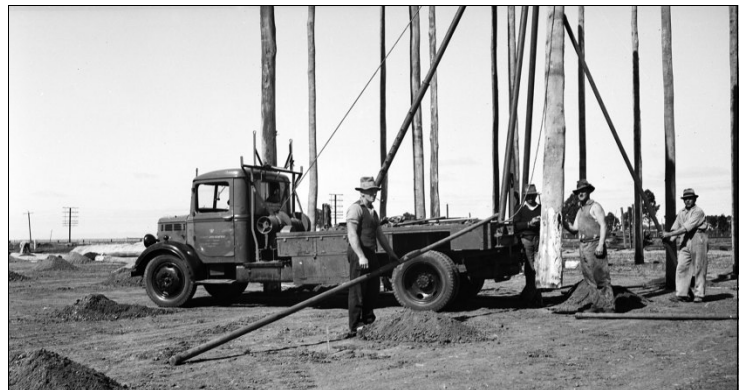
Erecting the Stick Shed poles using a crane truck, 1941. Ph: Culture Victoria.
