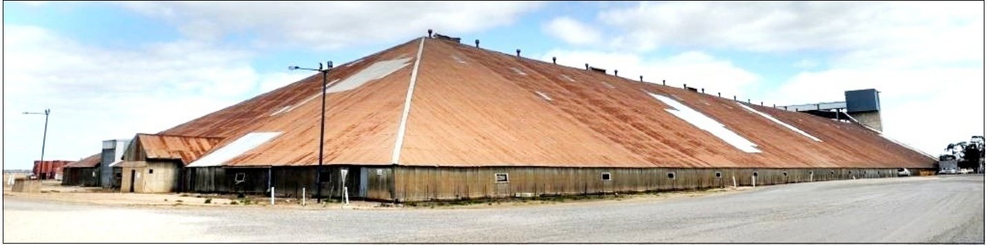
The Murtoa Stick Shed in 2013, viewed from the north-east. Photo: Wimmera Mail-Times.
