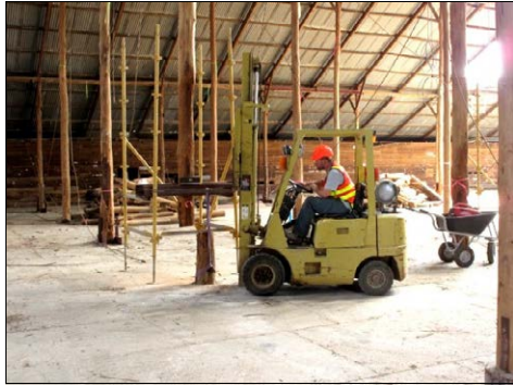
Pulling a rotten pole stump with a forklift. The upper pole has been moved aside & is held by scaffolding. Photo: Martin Zweep, January 2011.
