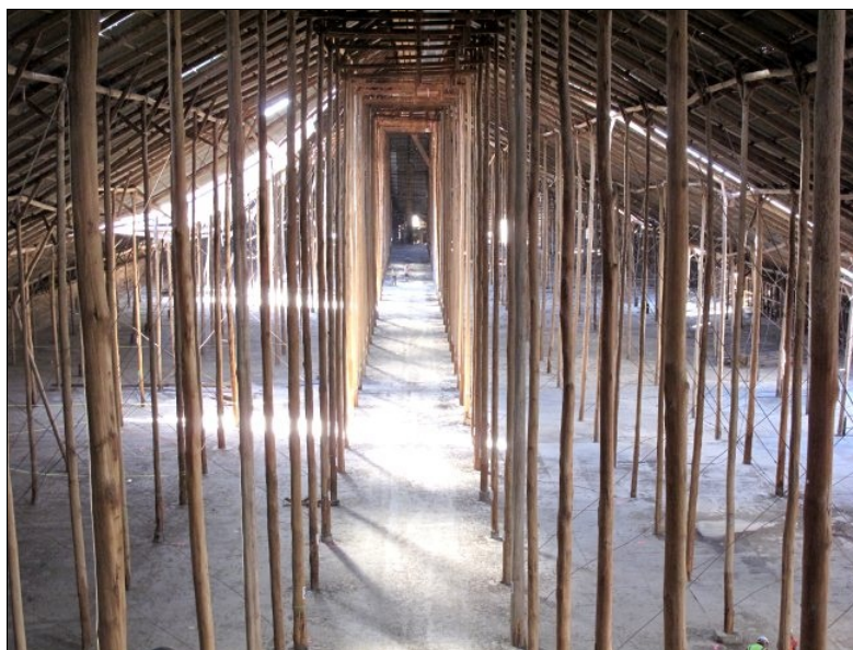
ABOVE: The interior of the Stick Shed in March 2009, before repairs began. Note the large hole in the roof at left. Photo: Martin Zweep, Heritage Victoria.
