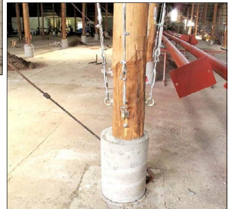
Repaired pole on its new concrete footing, showing diagonal bracing & the lower attachments of the bow trusses. Photo: Heritage Victoria, 2011.
