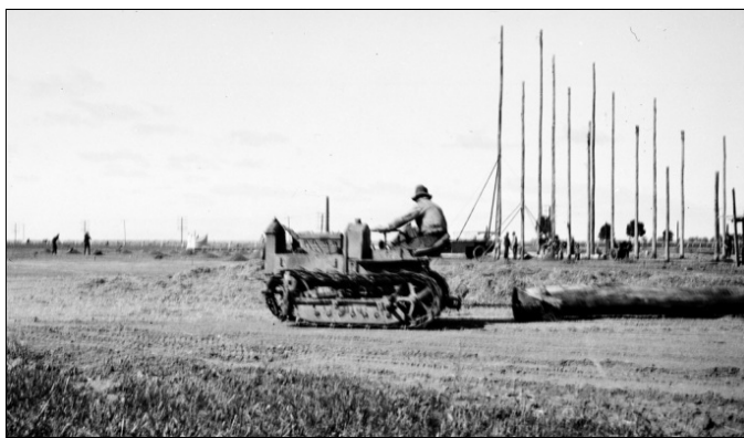
Dragging poles into position with an early caterpillar tractor, 1941 Photo: Culture Victoria.
