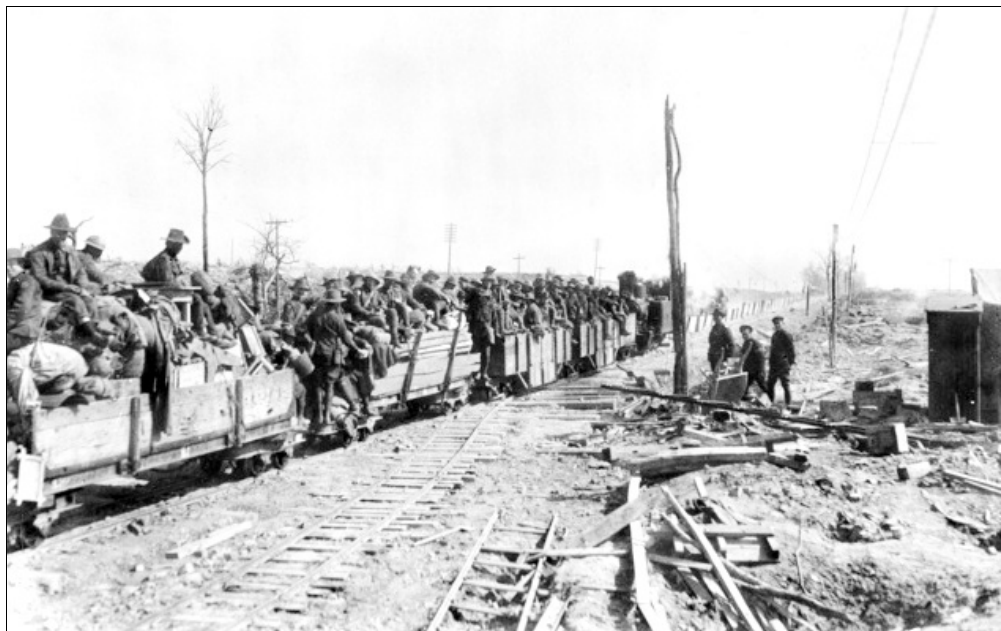
Soldiers from Australian 4th Pioneer Battalion moving behind the lines on a light rail train, around Warlencourt on 19 April 1917. This is the only image found of Australian soldiers engaged with Light Rail construction on the Western Front. Source: AWM Image 00468.
