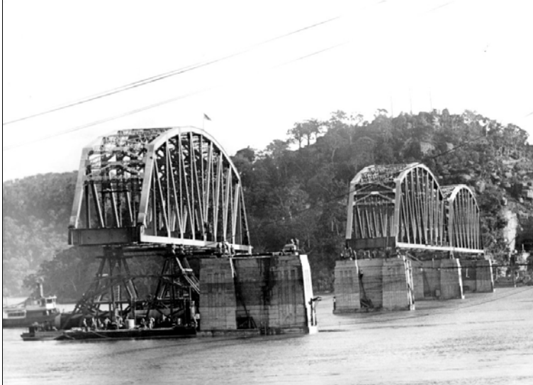
27 February 1944 - Span 3 of the bridge about to be fitted between its piers. Is that CCE Fewtrell standing on the centre of the bottom chord of the truss? Probably. Source: ARHSnsw RRC 47326.
