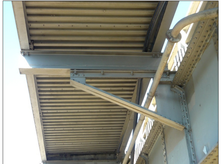
The footway on the downstream side. The rivetted brackets date from 1937. The superimposed steel section and the concrete slab are modern.
