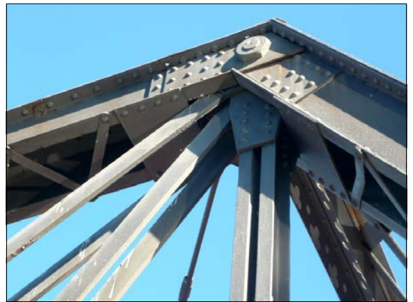
A pin joint at the top of the raking end post on the bridge. The pin connects all the members, including the raking end post and the top chord. Note the two diagonals connected to this point.
